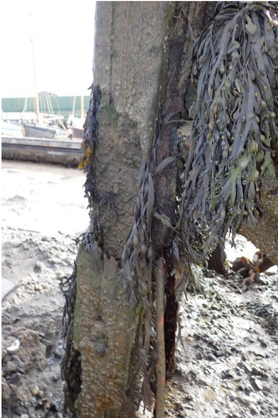
Fig 21 – Dolphin 3 loss of section of timber rubbing rail and poor condition of connection bolt
