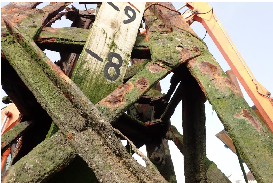
Fig 18 – Dolphin 3 typical condition note hole in diagonal bracing member
