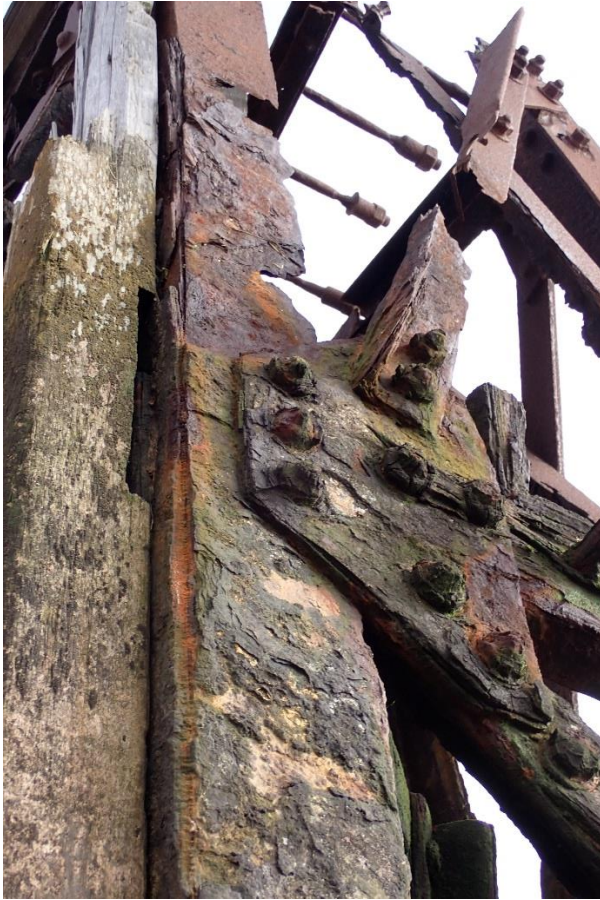
Fig 15 – Dolphin 3 above high tide line note deterioration of connections
