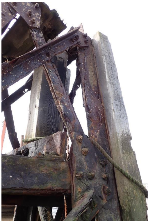
Fig 8 - Upper section of Dolphin 2 (note extreme loss of section)
