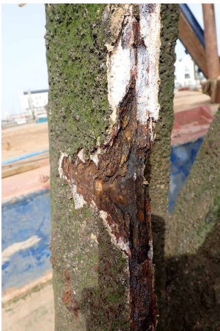
Fig 22 – Dolphin 3 condition of member under marine growth
