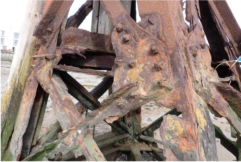
Fig 7 - Typical condition of joints on Dolphin 1 above high tide line
