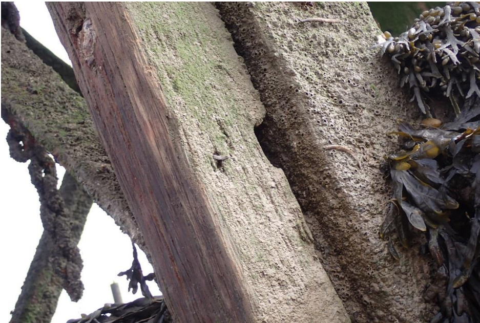
Fig 16 – Dolphin 3 typical condition of hardwood timber rubbing rail
