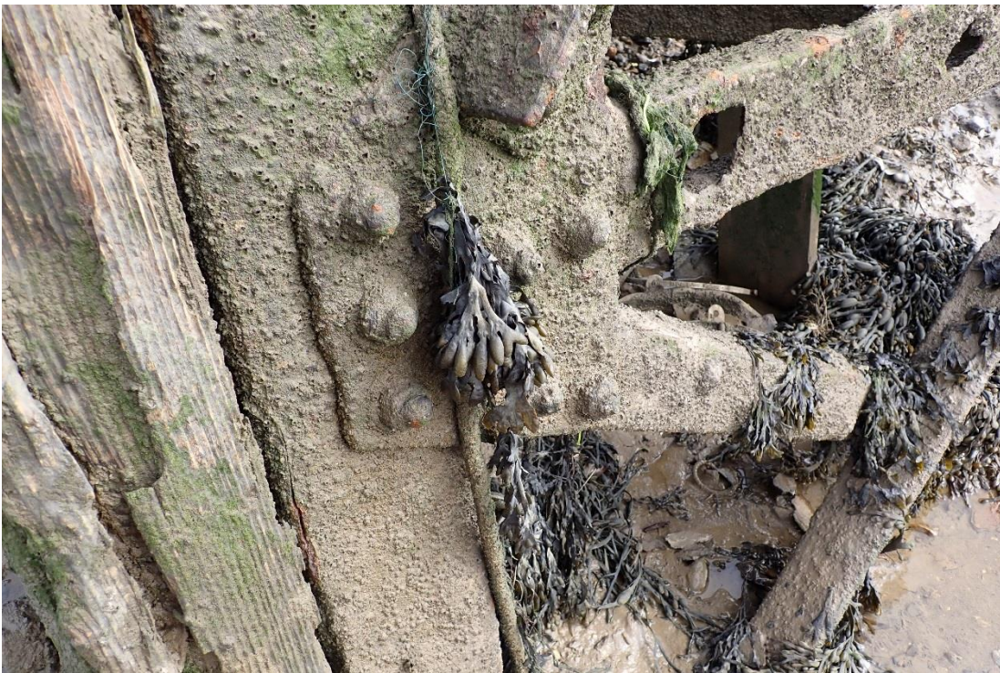
Fig 24 - Dolphin 3 typical marine growth below tide line
